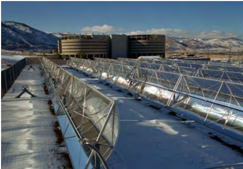
Figure F-4. This 4000 sf solar thermal system is similar to the size and type considered here.
