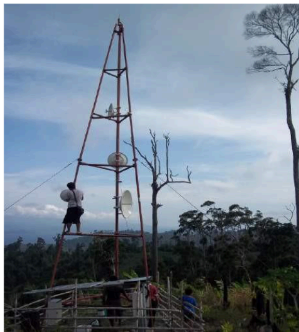
Figure 6: Wireless Network Tower in Sidangoli, West Halmahera.
